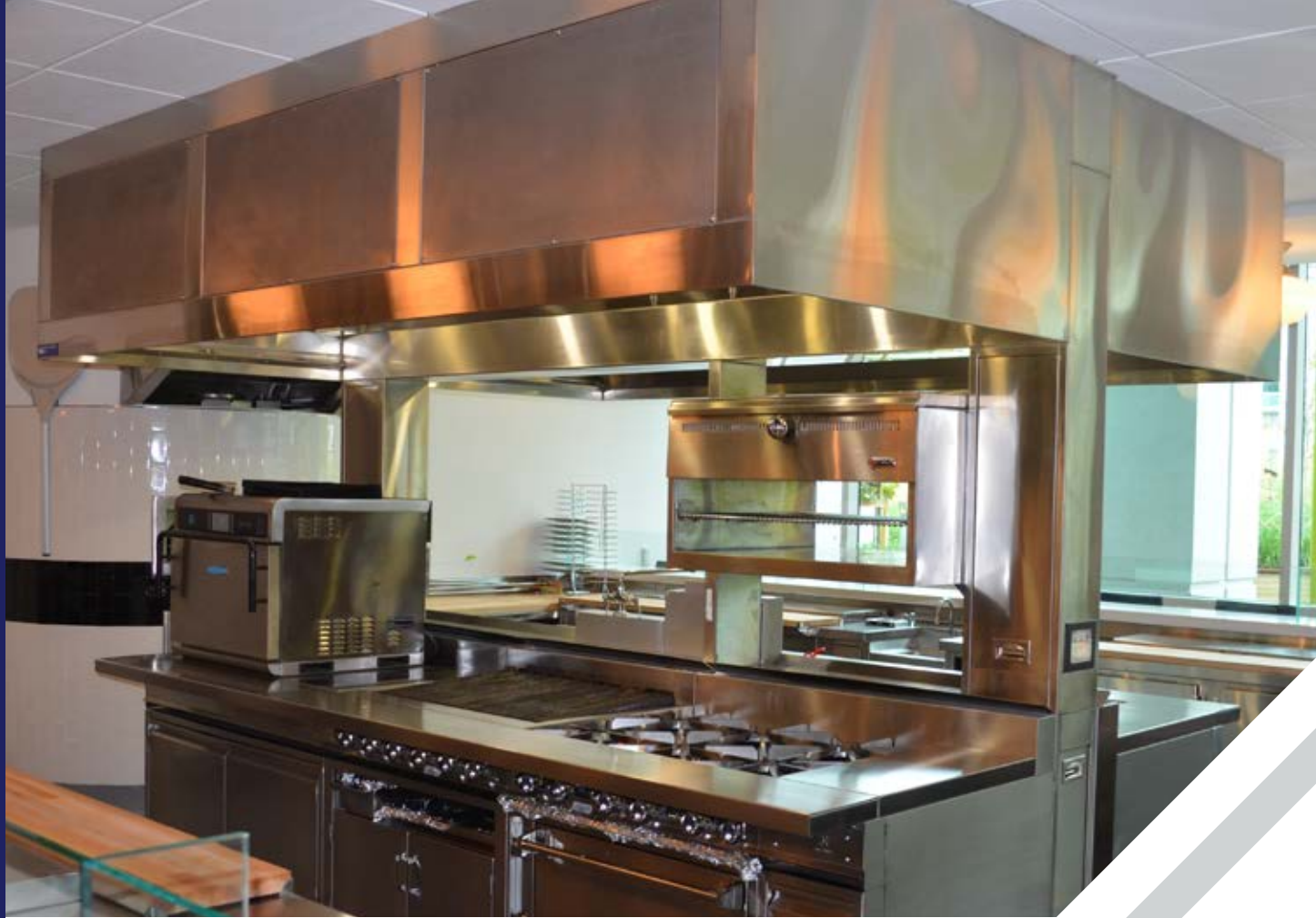
Human Machine Interface mounted to the side of the vertical wall. Vertical walls provide ideal locations for the installation of Demand Ventilation Controls and other electrical switches.
