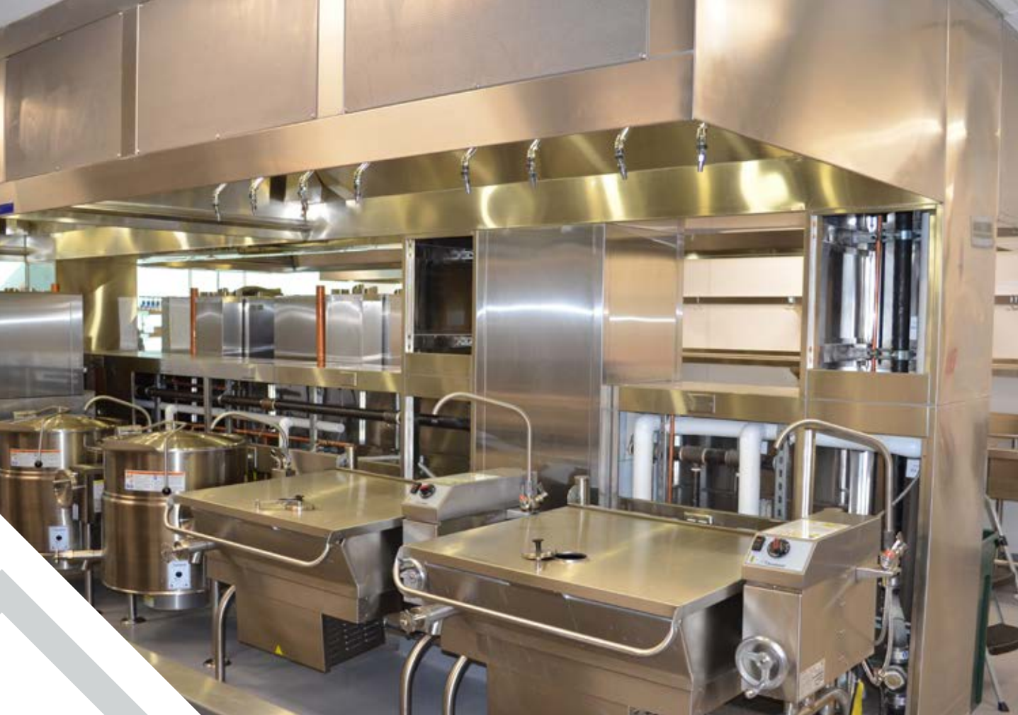
Utility Cabinet System with panels removed
