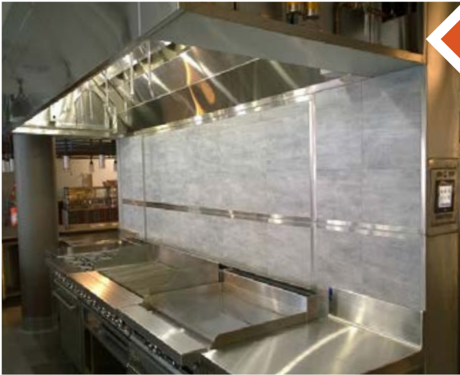
Utility Cabinet System with inset ceramic tiles
